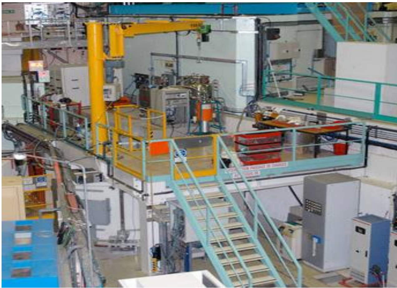
IN4c experimental facility
